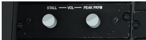
Figure 121. Stall Warning Control Panel
